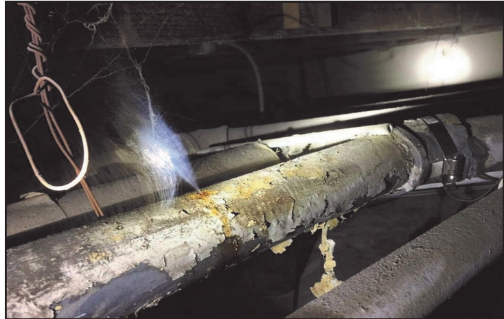
Image of a cracked hot water line at SAMS
